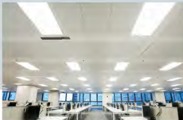
HSBC Data Centre, China Hong Kong
